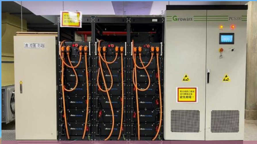
Taipei City Hall Energy Storage System
