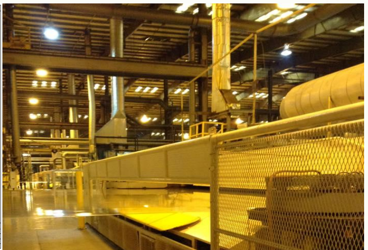
The place mount air curtain system.
